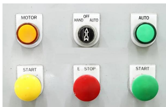
Figura 1 – Painel de Controle
