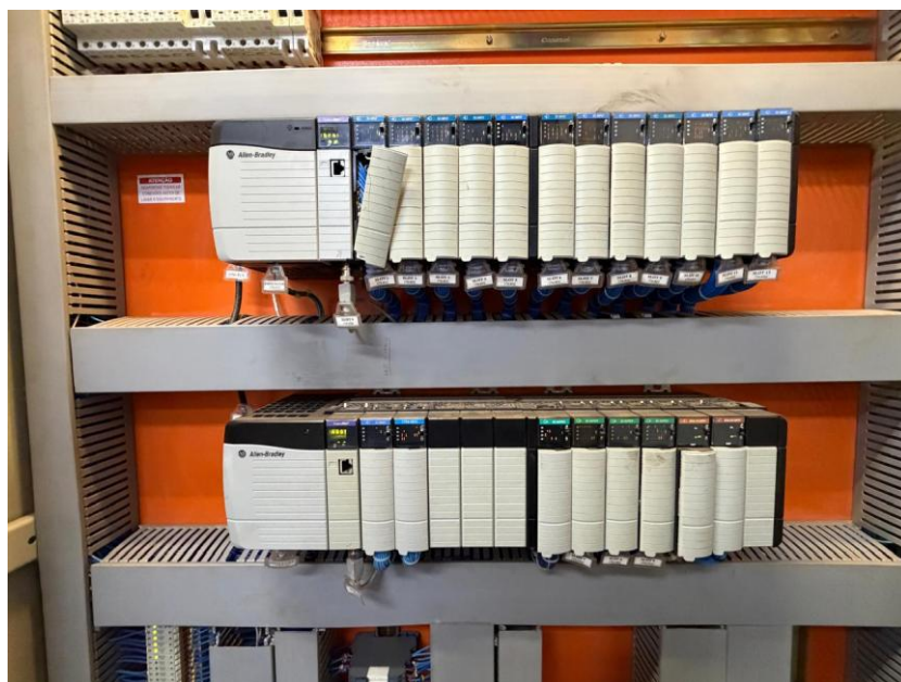
Figura 15 - CLP CompactLogix Instalado in loco
